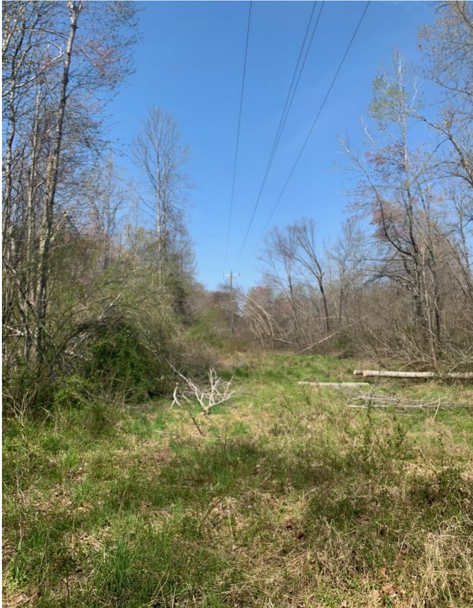
Figure 16. Example of Densely Overgrown ROW
