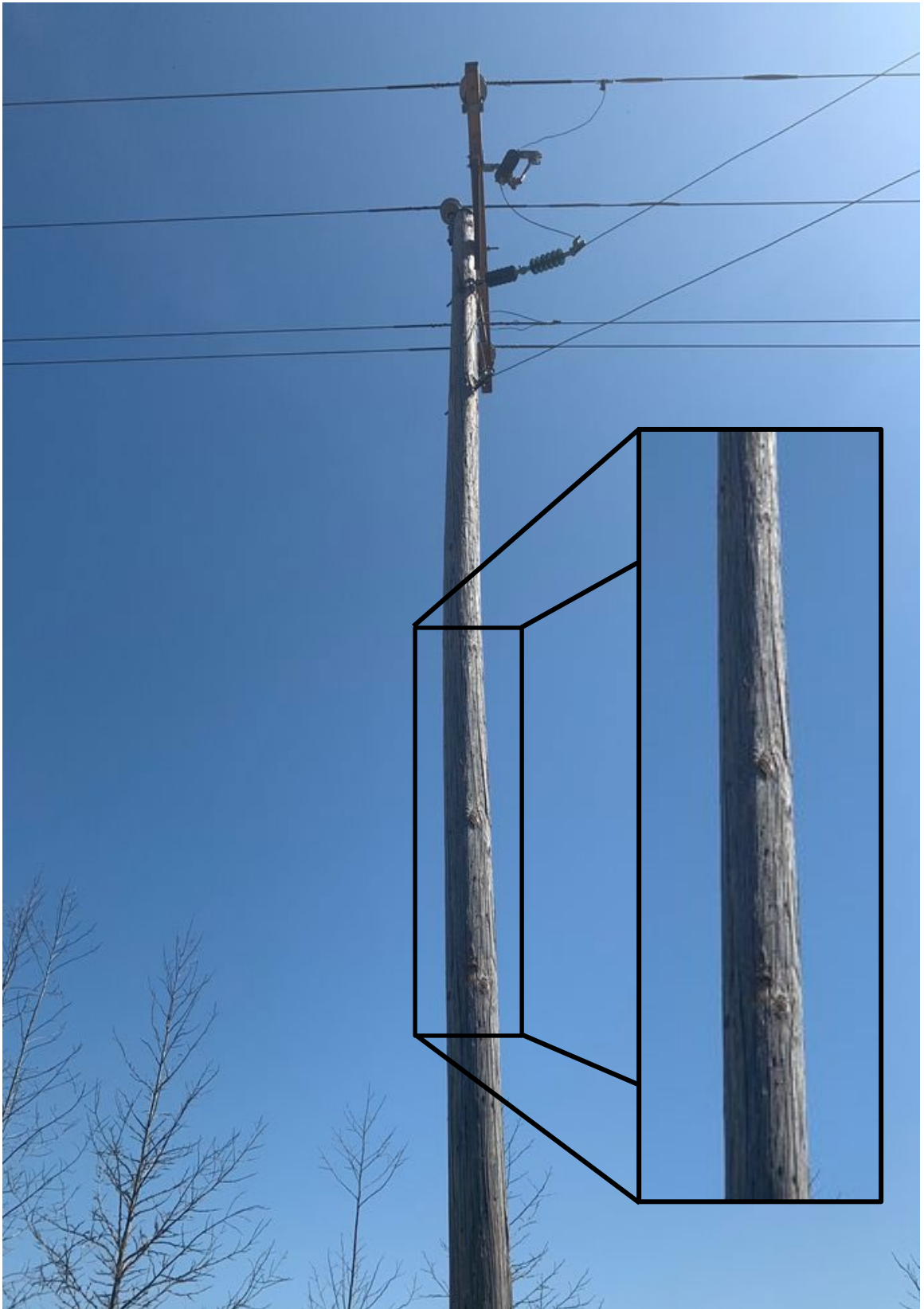
Figure 19. Pole with Wildlife Damage and Shellrot
