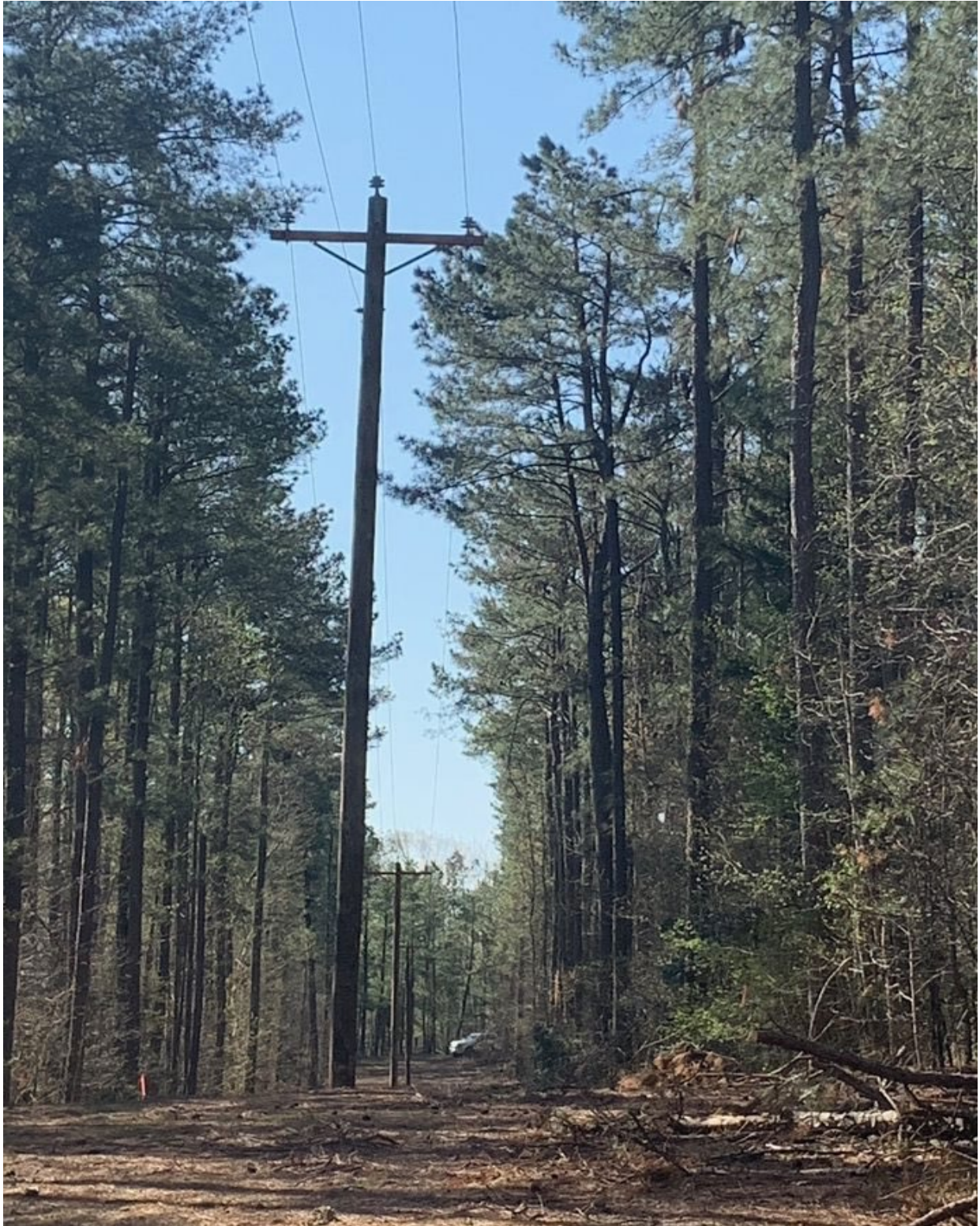
Figure 13. Limbs Overhanging Previously Cleared ROW
